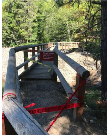
Left: Pedestrian Bridge on Lost Creek Lake Trail closed due to failing bridge support gabion
